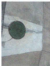
lift station 9"x6'
