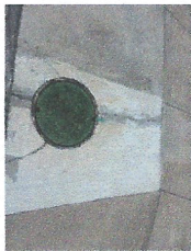
lift station 9"x6'
